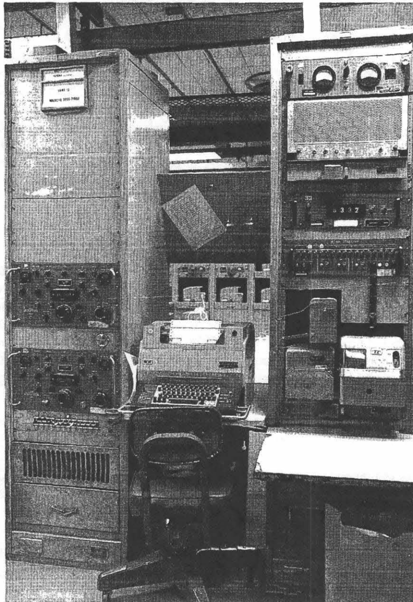
AG-22 - Configured Morse Position at USA-57, Clark AB, Philippines. (R-390 receivers are in the left-hand rack; MOD-35 in the center; and tape unit on the right)
